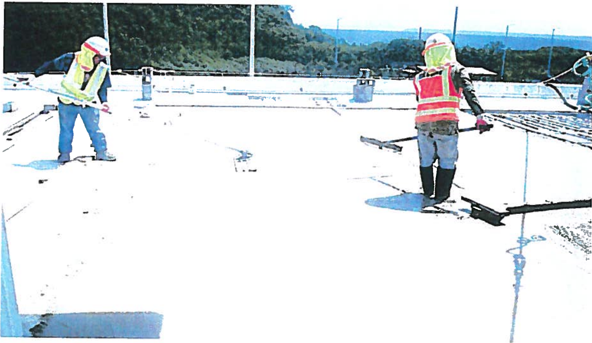
Construction workers poring and spreading cement on Port roof. Photo courtesy of the contractor
