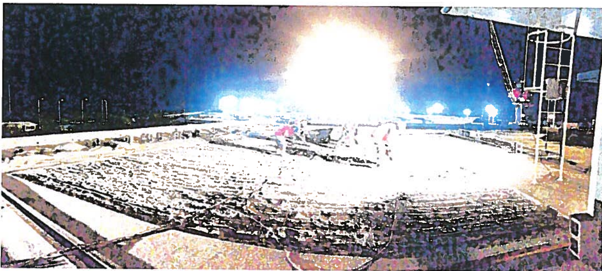
Employees from BBR Micronesia working late into the evening on roof repair of the Admin Building. Photo courtesy of the contractor.
