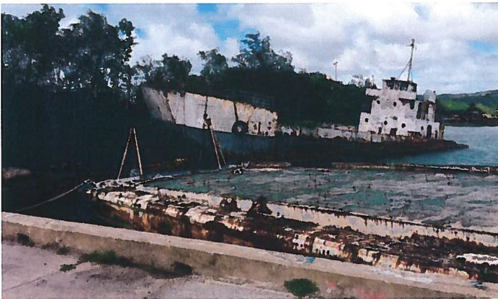
Work in progress in the removal of the Guahan I vessel and barge berthed at the Port F-6 pier.
