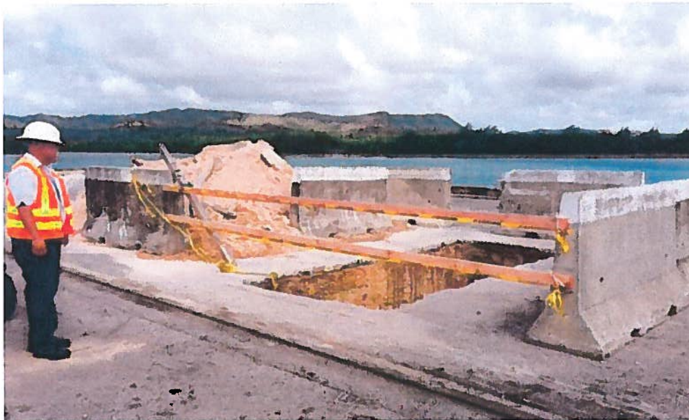
DGM Administration & Finance Alfred Duenas inspects the excavation for the pavement repair of the leaking waterlines.
