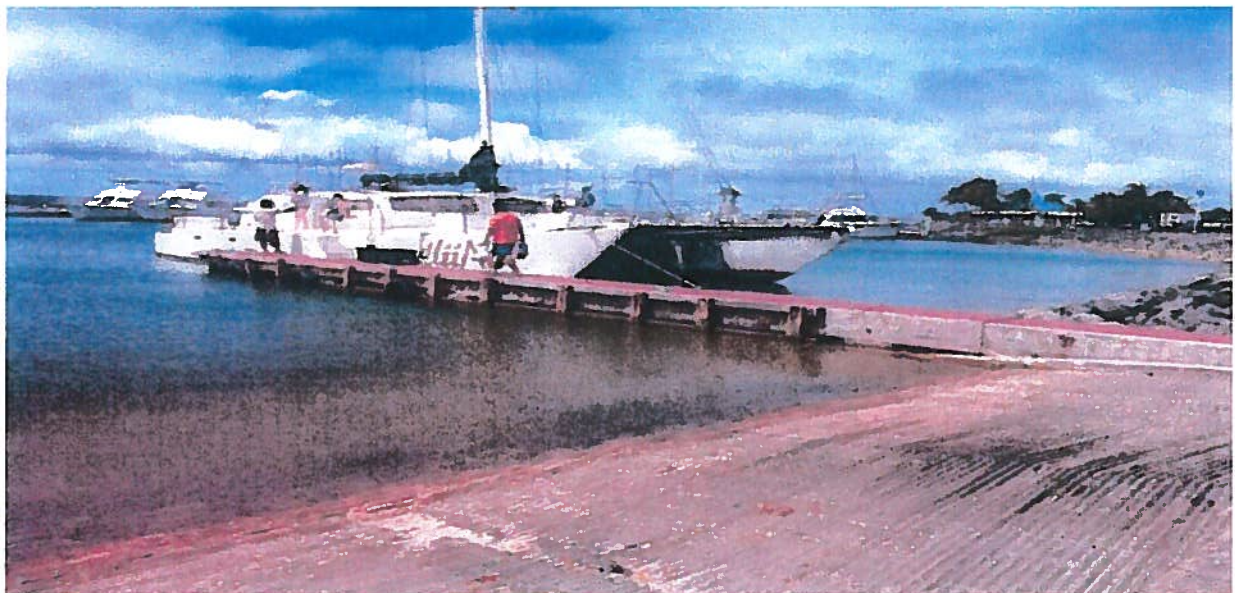
The Port's Planning Division is currently pursuing additional funding from the Department of Agriculture Sport Fisheries Boating Access Grant to address repairs to the second Cat Walk ramp displayed in the above photo.
