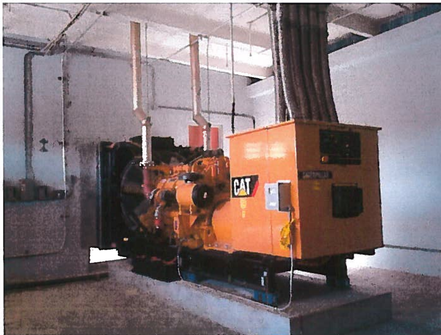
Installed 725KW Prime Power Generator at LC-4.
