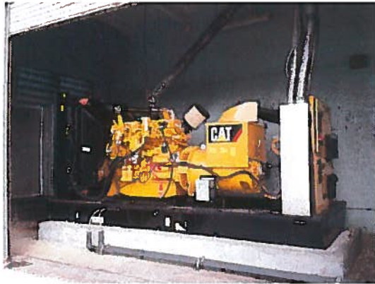
Installed 455KW Prime Power Generator at LC-1.
