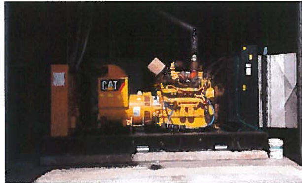
Installed 455KW Prime Power Generator at LC-2.
