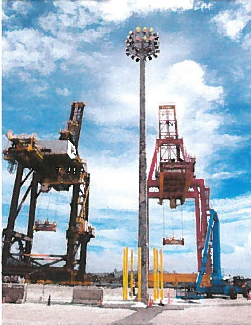
High Mast Lighting in Port Yard.
