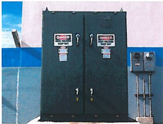
New LC-4 Metering Cabinet
