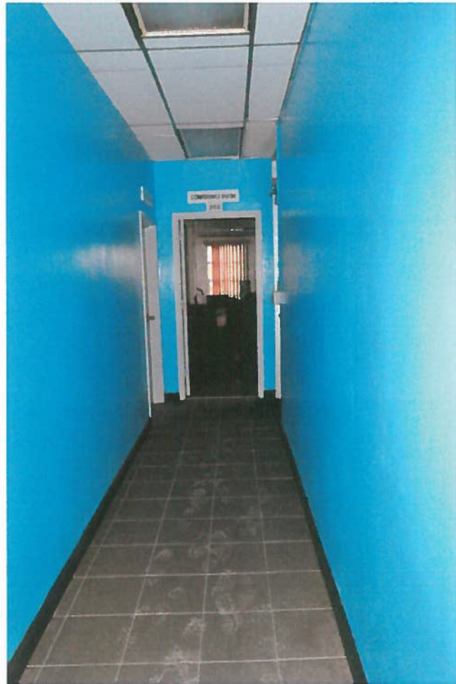
June 2, 2015: 2 nd floor hallway covered in soot.
