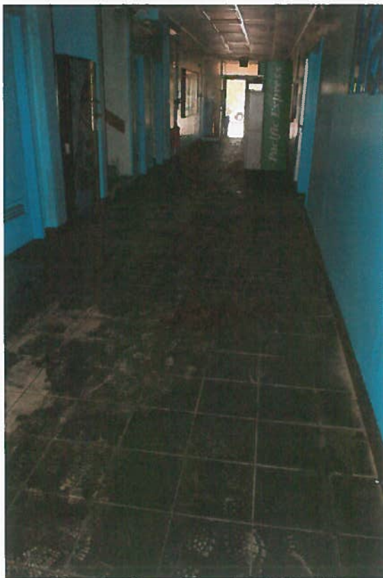
June 2, 2015: 1 st floor hallway covered in soot.
