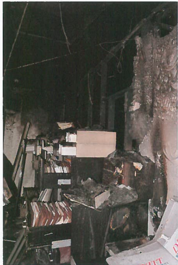
June 2, 2015: HR personnel files listed as top priority in the restoration efforts.
