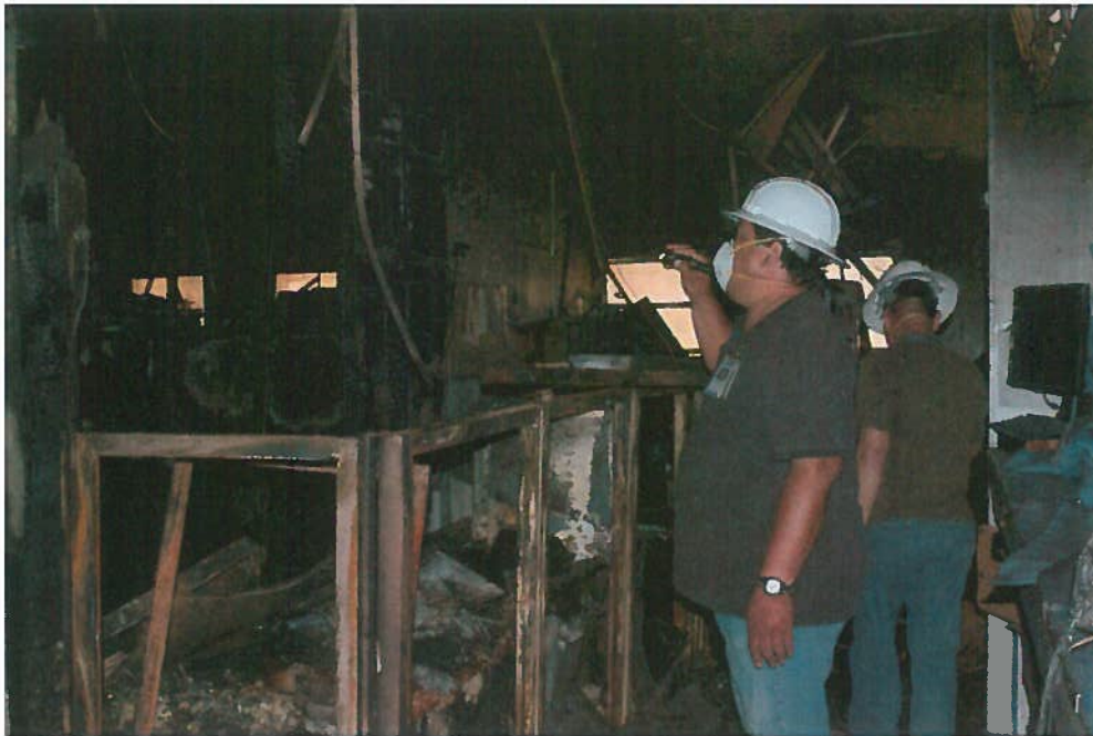
June 2, 2015: Port Management Assessment Team inspects fire damage of Customs & Quarantine Office.
