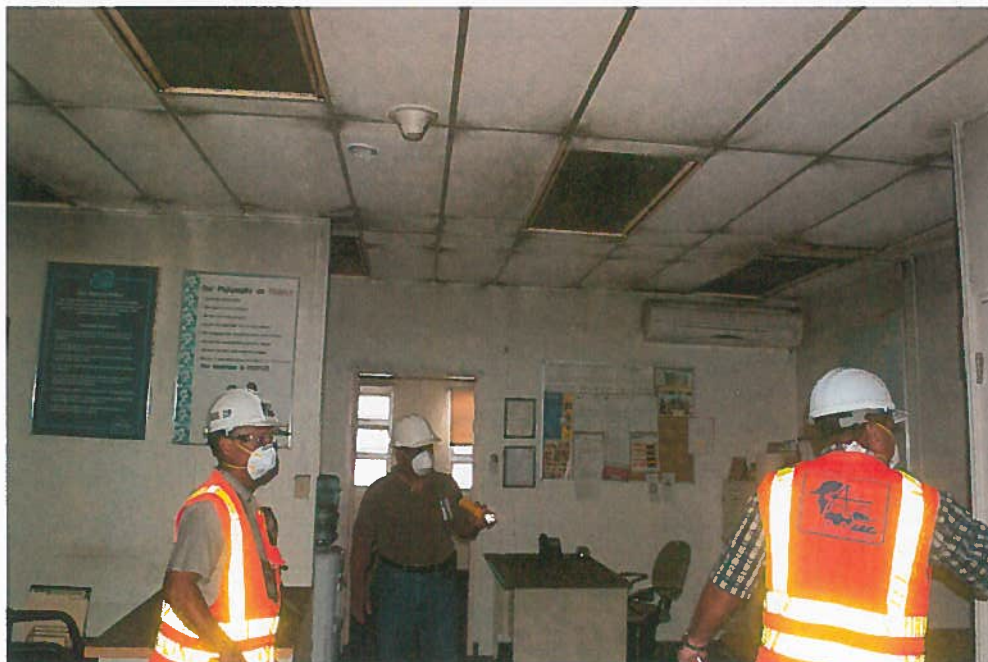
June 2, 2015: Port Management Assessment Team inspects smoke damage in the CTSI office.
