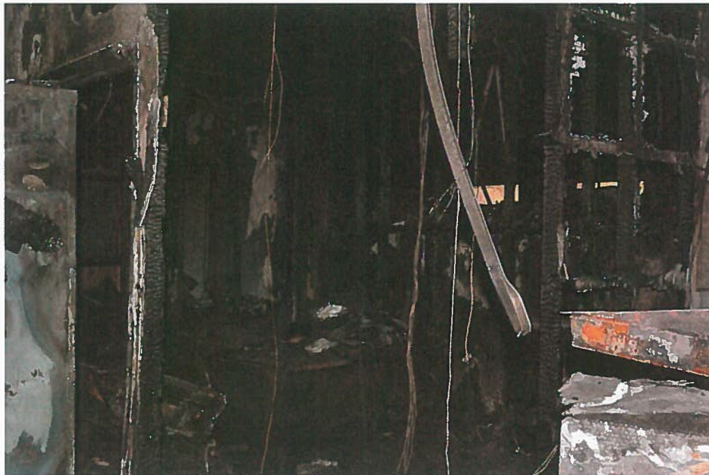
June 2, 2015: Customs & Quarantine Office total damage as a result of the fire.
