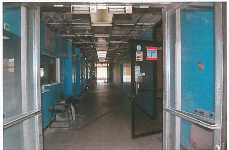
June 30, 2015: Post-cleanup efforts to the 1 st floor hallway covered in smoke damage.
